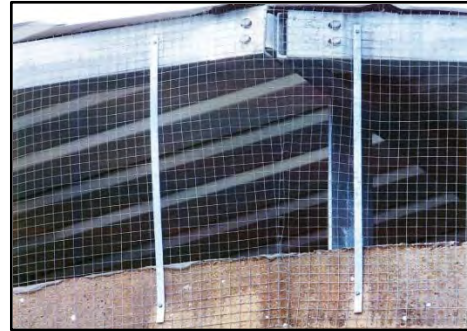
Photo 4 – Deficient reservoir roof design
