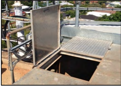
Photo 1 - Service reservoir hatch left open
