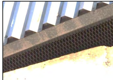
Photo 5 - Large mesh openings on reservoir
