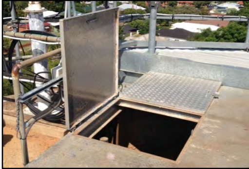
Photo 1 - Service reservoir hatch left open
