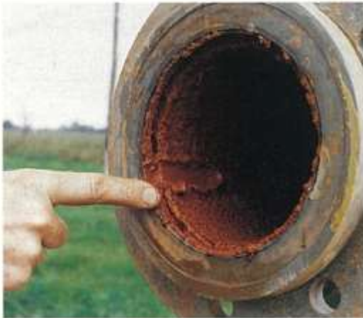
Slime build up inside delivery pipe.
