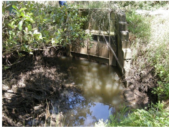
Figure 36. Downstream drainage constrained by mangrove and sediment build up, but floodgate is still able to function
